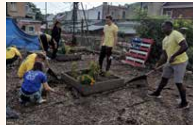
△ As part of the renovation, employees helped paint the exterior and plant gardens around the building.
